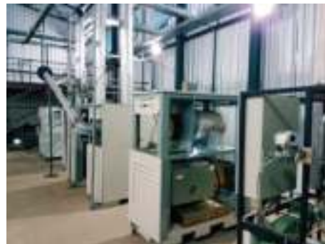
Gas microturbines and chiller
